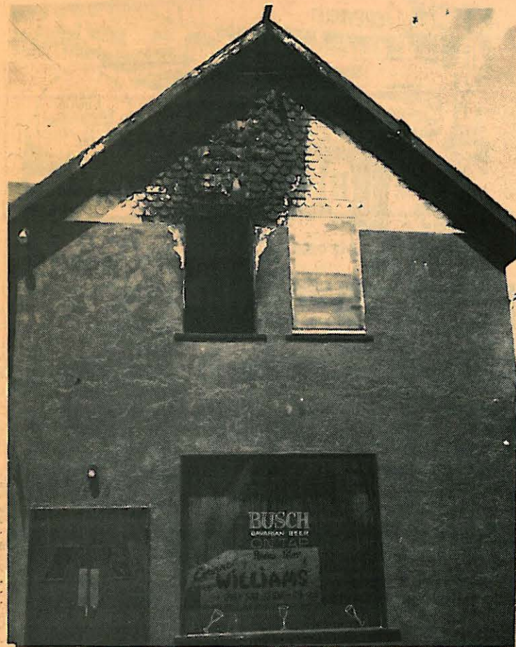
THE EXTERIOR OF THE LAKESIDE HOTEL FOLLOWING THE SATURDAY NIGHT FIRE WHICH STARTED IN A MATTRESS. THE FIRE WAS QUICKLY BROUGHT UNDER CONTROL BY THE LAKESIDE FIRE DEPARTMENT.
